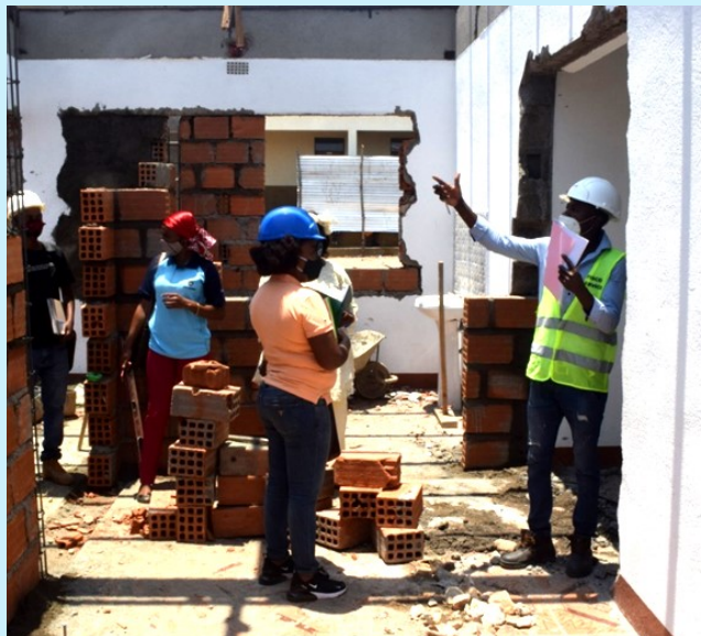
Provincial Assembly members visit the construction works for the Health Center sanitary block in Meponda.
